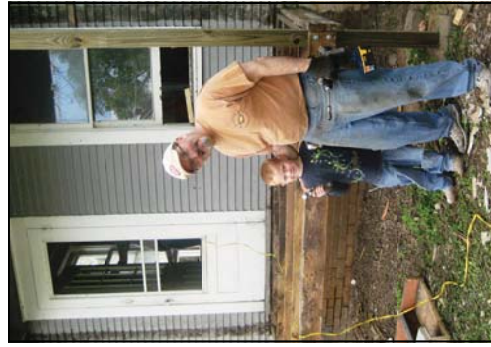
Keegan Toule (left) and Brad Hager (right) work on rebuilding the back porch of the donated home.
